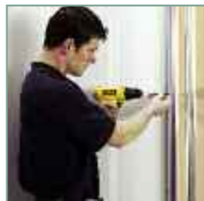
The door is finally secured by drilling through the wall channels into the door frame and fixing with screws.
