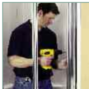
The wall channels are then slotted onto the door and screw fixed to the wall.
